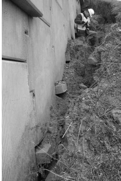
Figure 5-16. Example of surface flow erosion at the bottom of an MSE wall.
